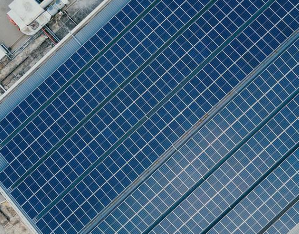
Solar system at the factory
